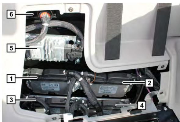
Figure 26: Control units behind the right passenger seat
